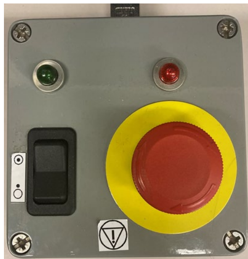
Figure 12. Remote System Power Box: Genesis with Siemens
