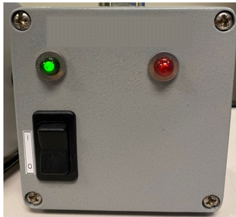
Figure 10. Remote System Power Box
